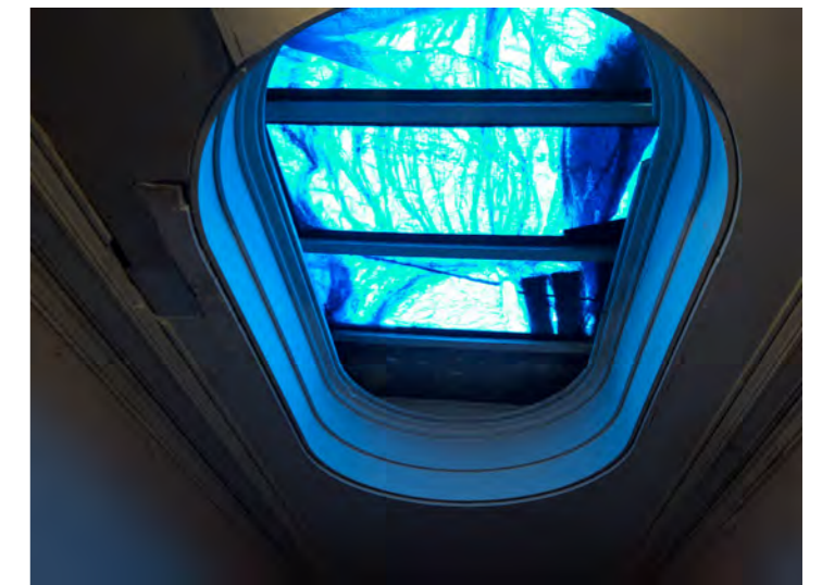
A broken / missing skylight over the secondary staircase
