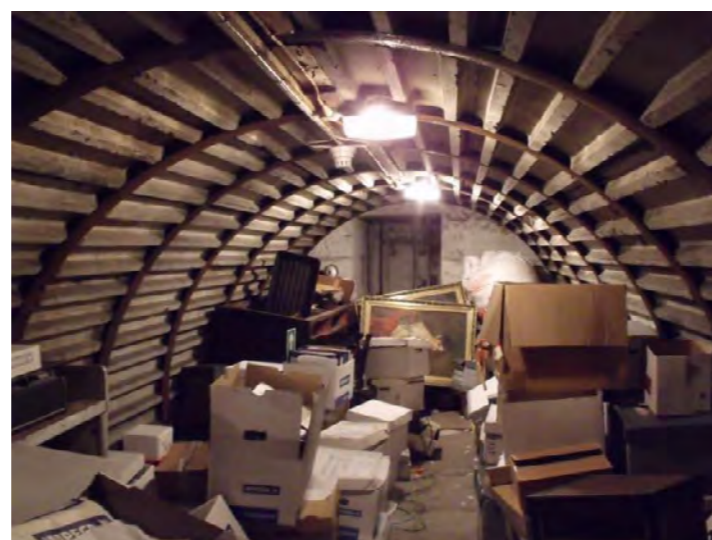
Image from 1991 showing the steelwork in the basement of the former bomb shelter.
