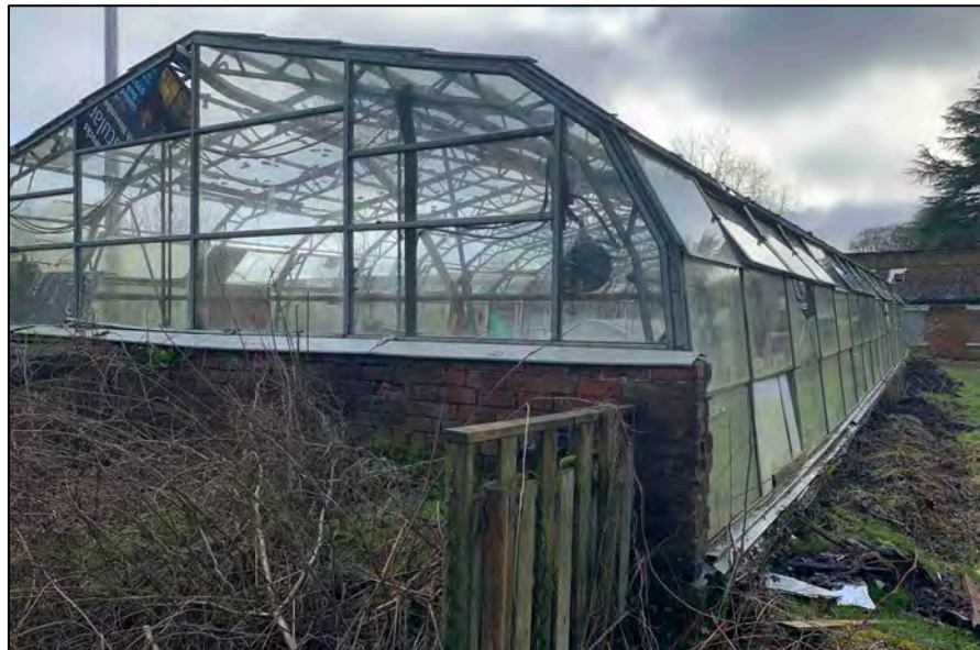
Appendix 2.5: View of Greenhouse to north of Bothy Range; note early brick stub walls
